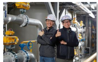
Wastewater treatment facility
