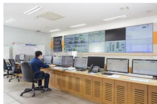
24-hour monitoring room for wastewater treatment
